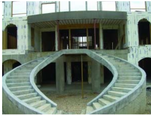
Bartley Corp. created a suspended half-moon staircase that was mostly supported by the top landing and steel reaching from the patio to the back of the residence.
