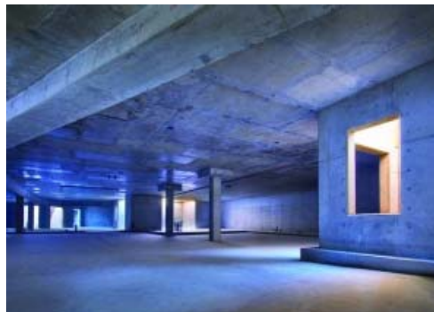
Ekedal Concrete's winning Villa Del Lago project featured 60 corners and angles as well as a structural deck above the foundation.
