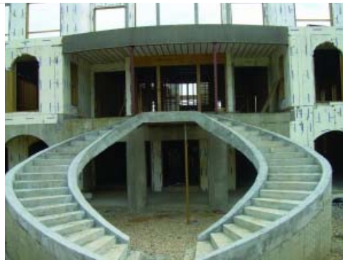
Bartley Corp. created a suspended half-moon staircase that was mostly supported by the top landing and steel reaching from the patio to the back of the residence.
