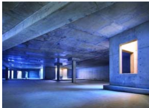
Ekedal Concrete's winning Villa Del Lago project featured 60 corners and angles as well as a structural deck above the foundation.
