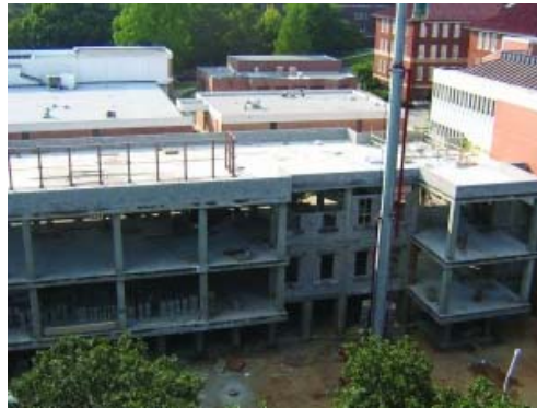
Action Concrete Contractors used four different forming systems for the walls, elevated columns and slabs of this dormitory addition.
